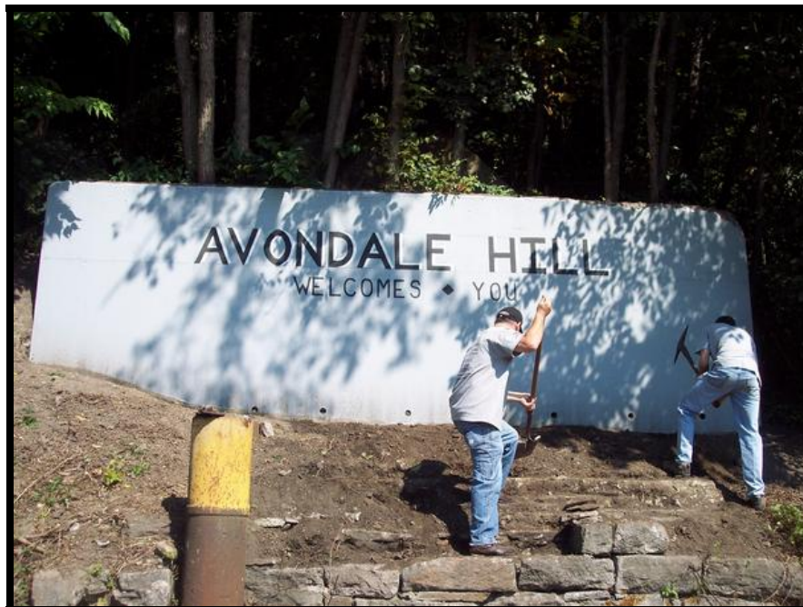
Robert (center) with shovel uncovering the historic masonry foundation block of the Avondale Mine Colliery pulley house structure and Zach Petroski (right) with pick in hand trying to level out a garden bed for the community garden. Note the 12” diameter borehole (left of center)
