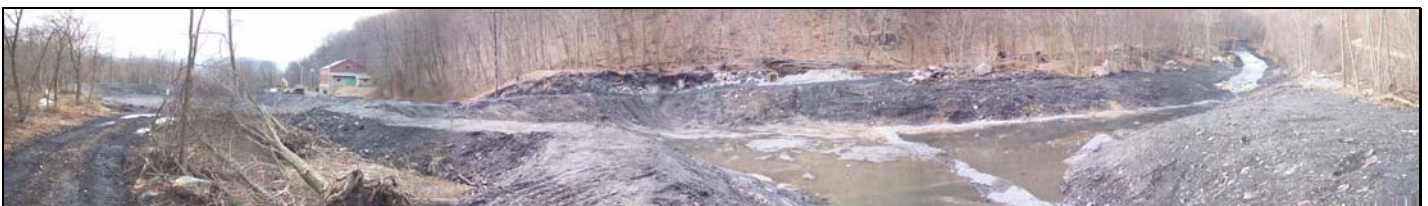
Construction of the Upper Settling Basin and diversion of AMD from the Lykens Water Level Tunnel, Dauphin County
